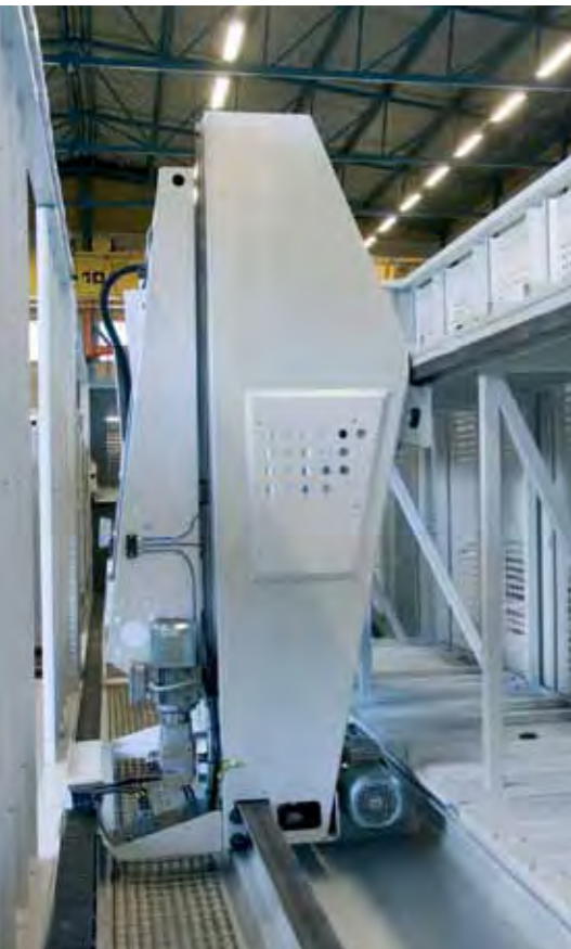
Storage view with stacker crane.
